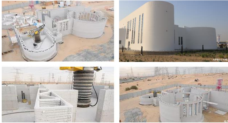
Figure 1.5. Apis Cor's 3D-Printing Machine was Moved About the Site Using a Crane to Re-Position it so it Could Build Different Parts of the Building [19]
